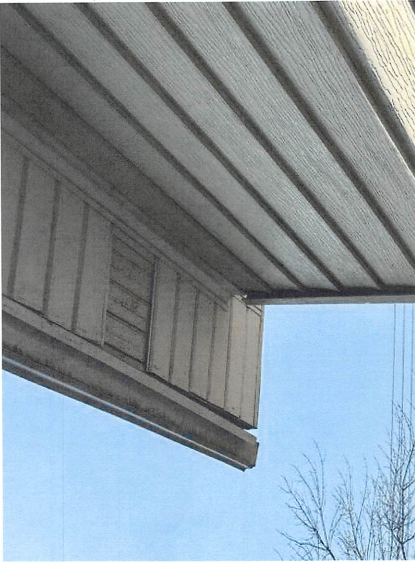
MISSING SOFFIT PANELS ON SW SIDE
