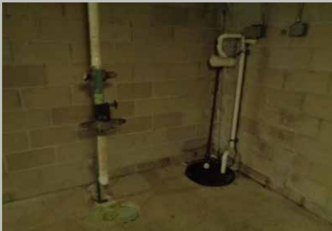
View of basement sump pump
