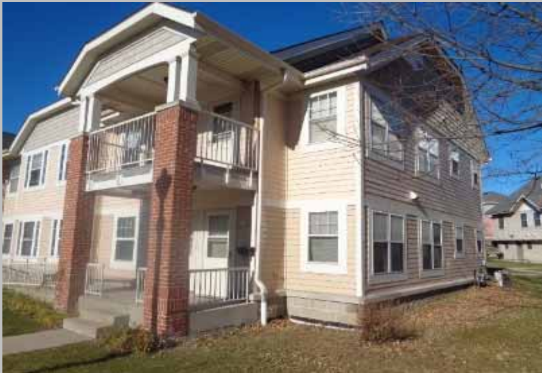
Additional view of trees encroaching on the building envelope at select buildings across the site (Non-Critical Repair).
