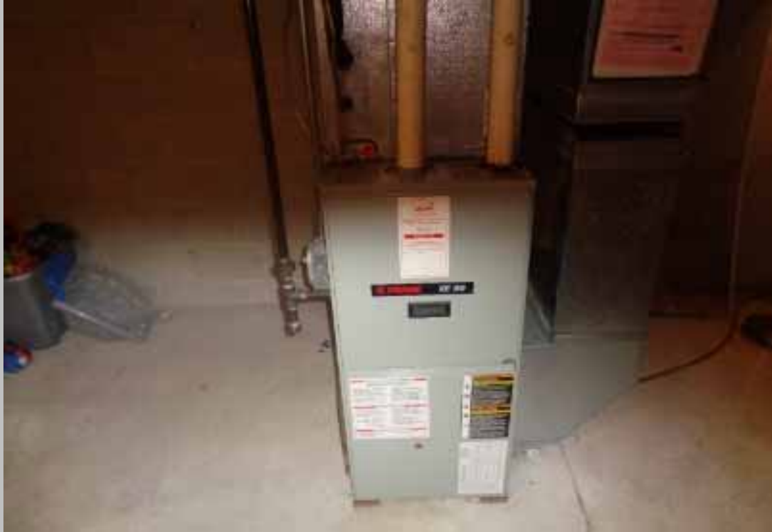
View of typical dwelling unit gas furnace.
