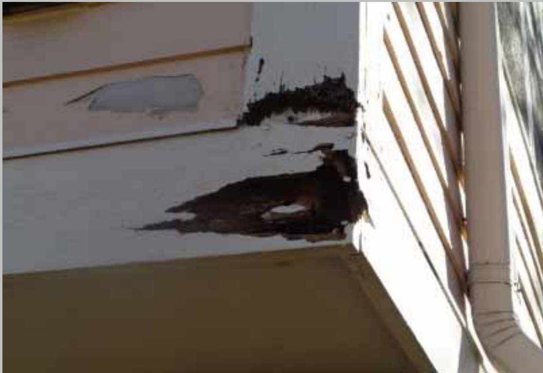
View of exterior trim with rot (Non-Critical Repair).
