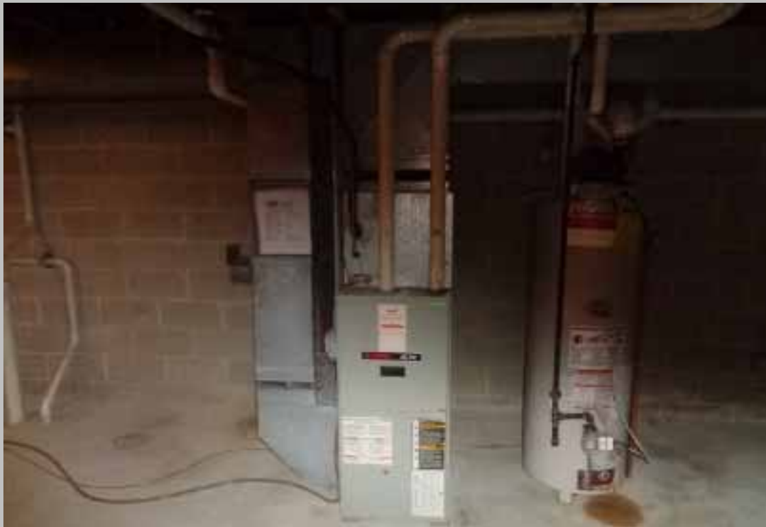
View of typical dwelling unit gas furnace and gas water heater.
