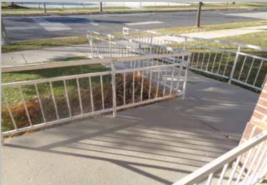
View of typical handicapped access ramp at ground floor units, with deteriorated concrete and oversized expansion gaps (Non-Critical Repair).
