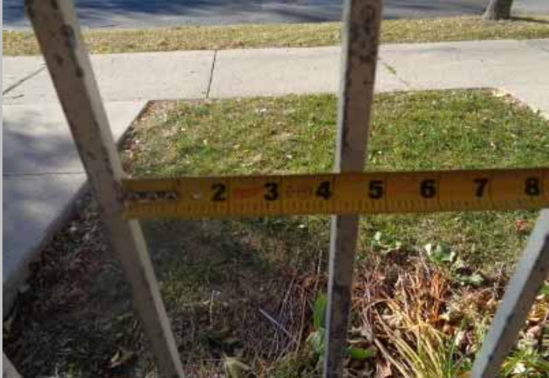
View of non-compliant (greater than 4-inches) metal railing balusters (Critical Repair).
