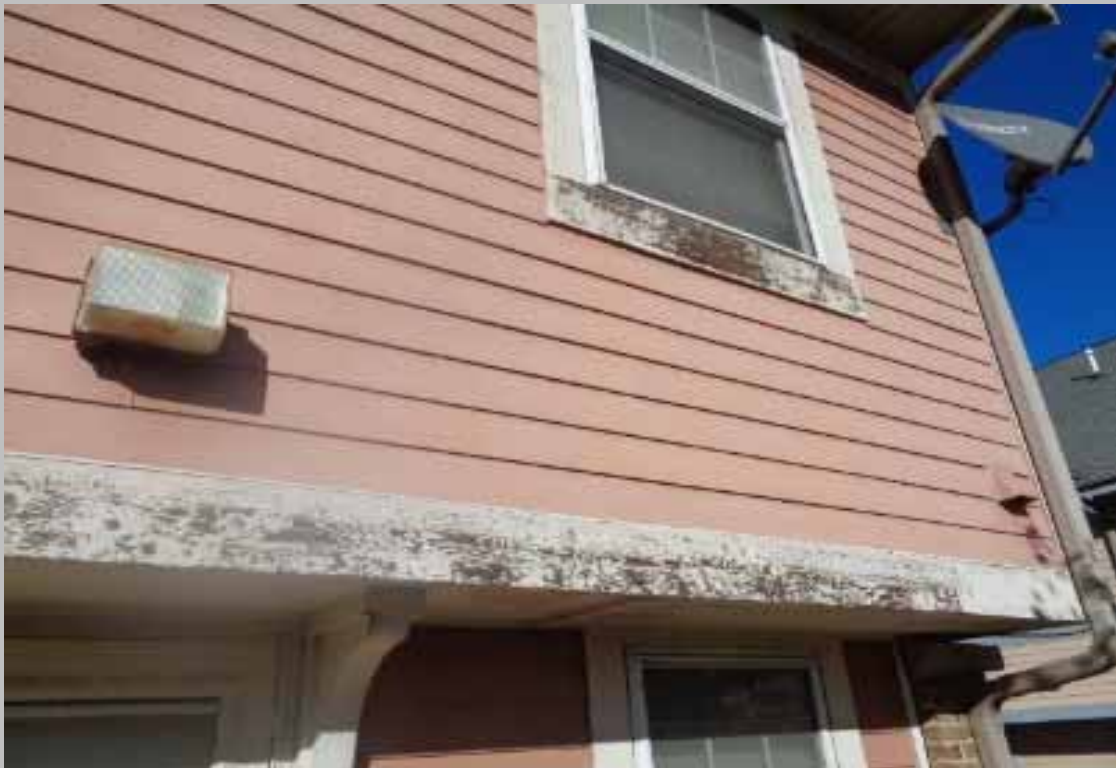
View of deteriorated exterior paint and trim observed at buildings throughout the site (Non-Critical Repair).
