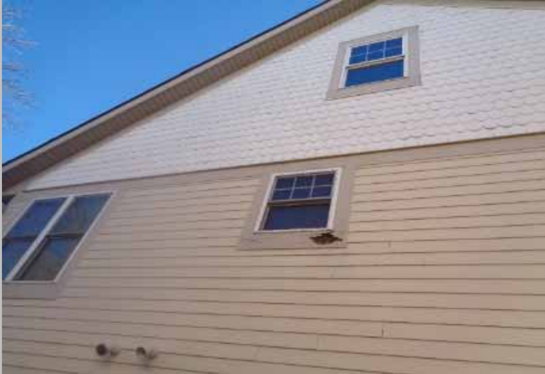
View of deteriorated exterior paint and trim observed at buildings throughout the site (Non-Critical Repair).
