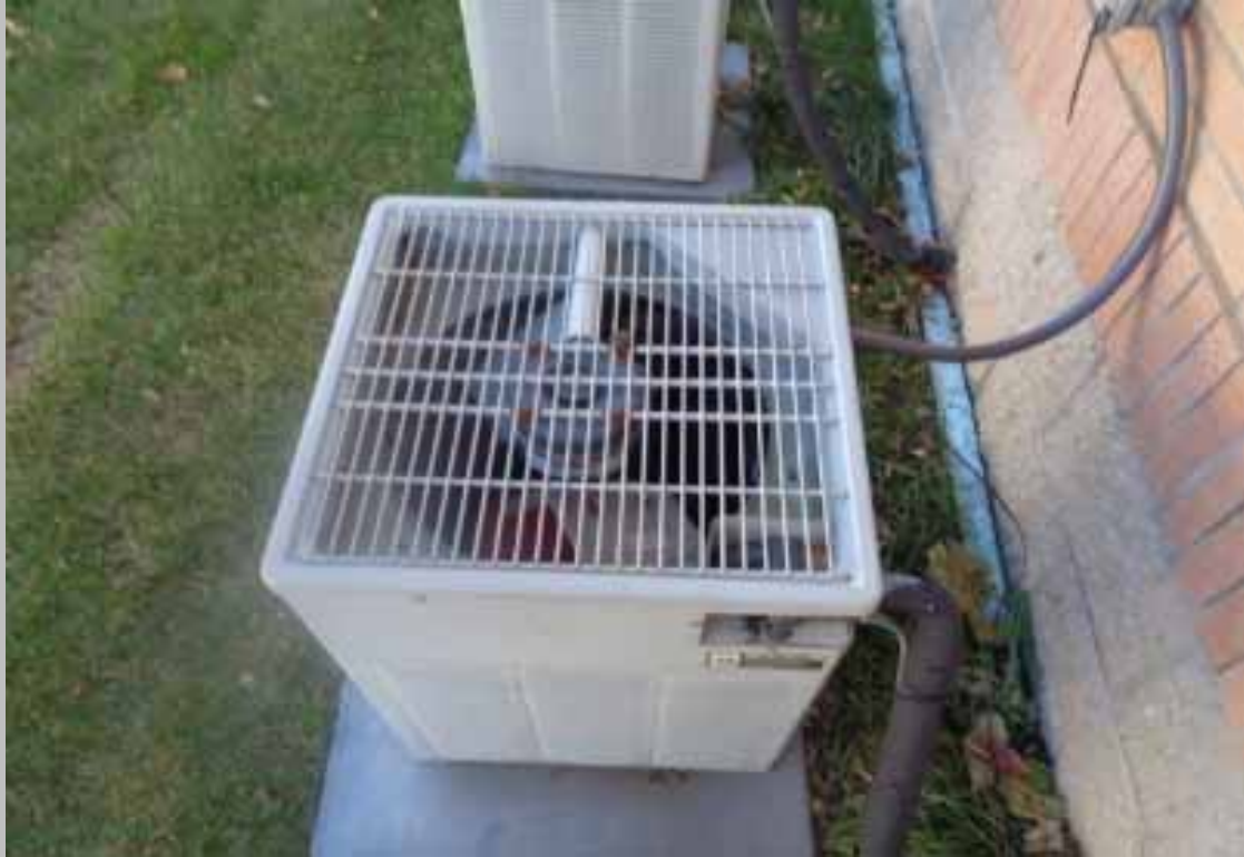
View of typical dwelling unit exterior condensing unit.
