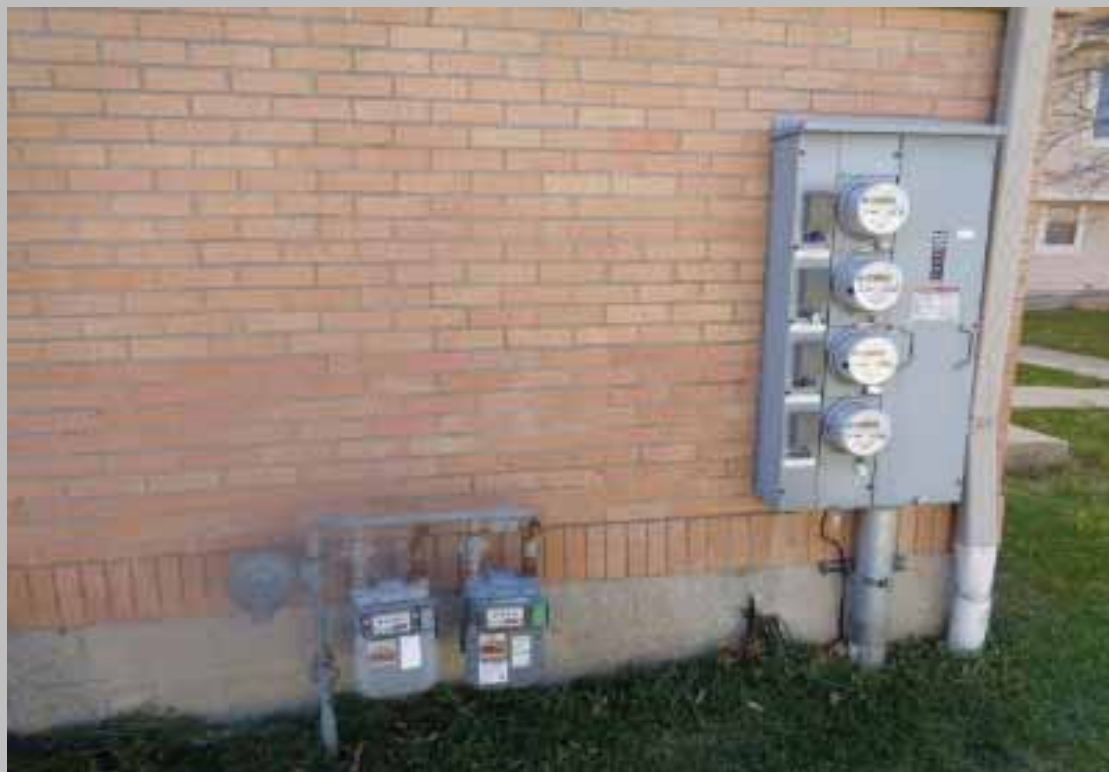
Gas and Electrical Meter
