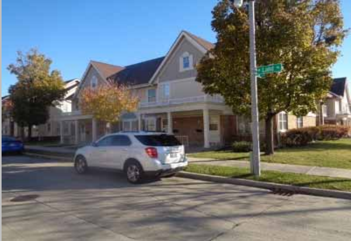
View of trees encroaching on the building envelope at select buildings across the site (Non-Critical Repair).
