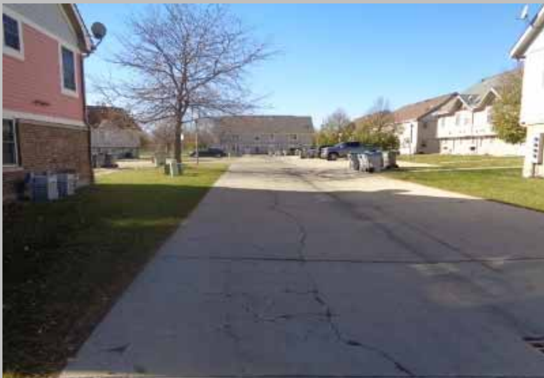
View of deteriorated concrete. (Non-Critical Repair).
