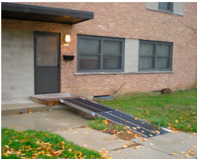
Design Deficiencies - Retrofits to Existing Units to "Accommodate" Accessibility
