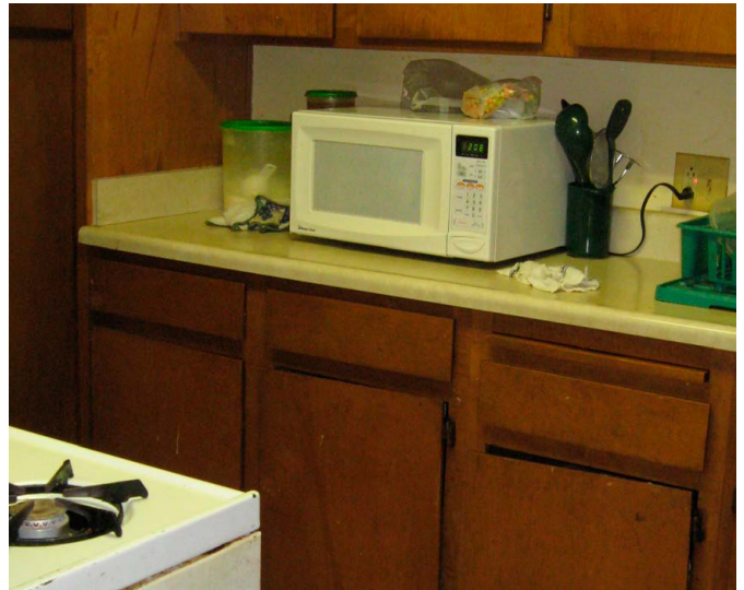
Design Deficiencies - Undersized Kitchens Compared to Current Standards
