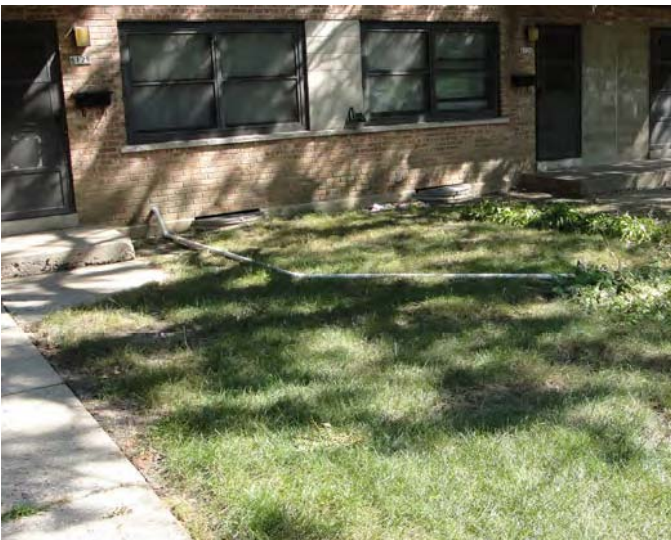
Structural Deficiencies – Ineffective Retrofit Discharge Pipes Create Hazards
