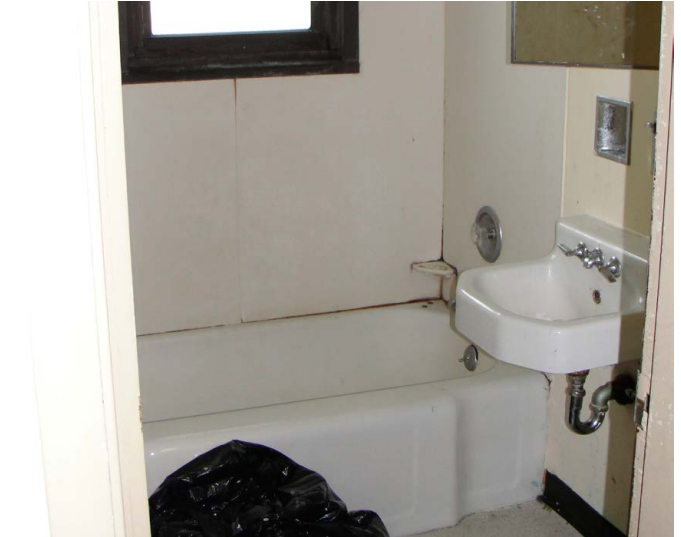
Design Deficiencies - Non-Compliant, Undersized Bathrooms
