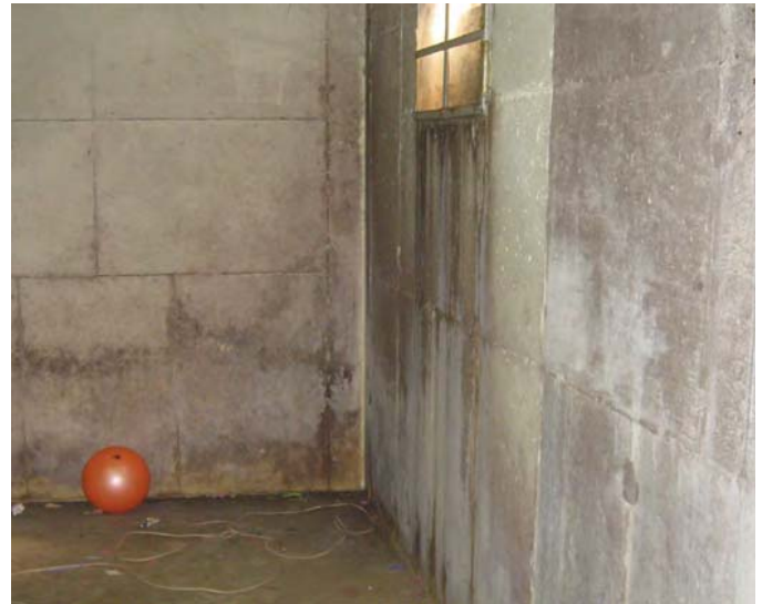
Structural Deficiencies – Poor Site Drainage Results in Flooded Basements and Mold
