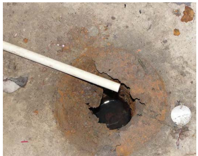
Structural Deficiencies – Unsafe and Unsanitary Conditions
